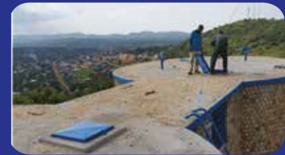
Twin Reservoir Tank
