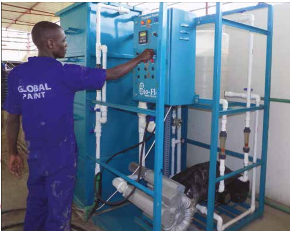
A water filtering process.
